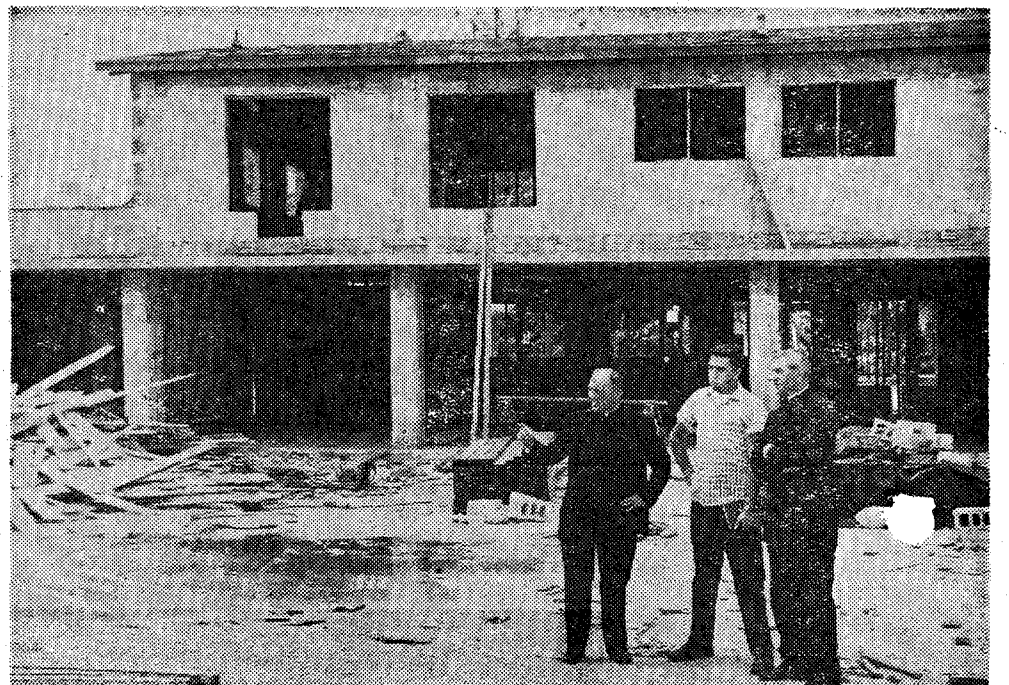
Construction of the new Catholic Student Center at the University of Miami, Coral Gables, was begun in June. Father John F. Monroe, O.P., left, chaplain, and Father Stephen B. Jur-
