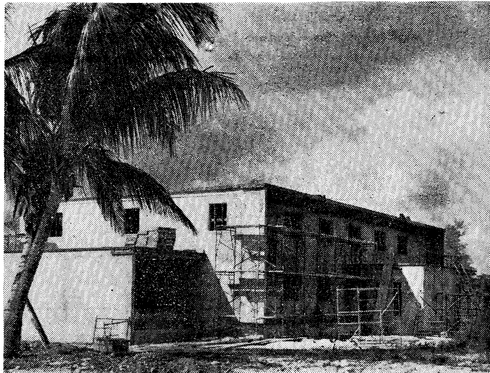
NEARING COMPLETION is the new faculty residence for Vincentian Fathers staffing the St. John Vianney Minor Seminary in Miami.
