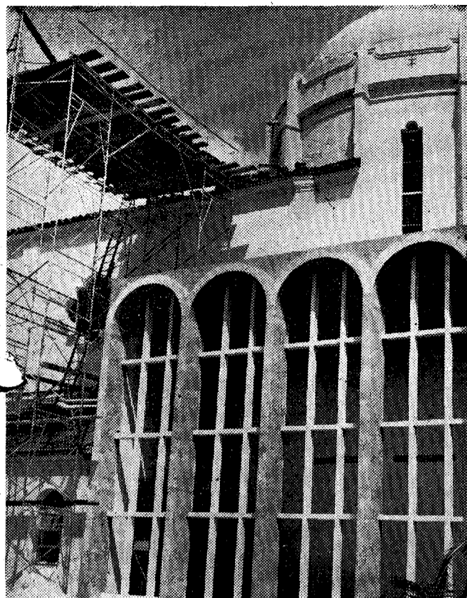
GRACEFUL ARCHWAYS in the Blessed Sacrament Chapel now under construction on the south side of St. Mary Cathedral are prepared for the installation of stained glass from Chartres.
