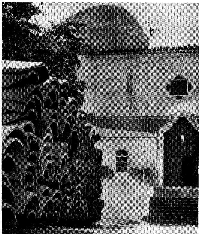
COLORFUL TILES are being laid on the roof at St. Mary Cathedral as work progresses rapidly on installation of stained glass windows in sacristy, sanctuary and nave of the church.
