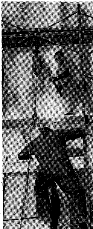
TWO TOWERS, each 30 ft. high provided support for the lifting of the giant console to the choir loft of St. Mary Cathedral.
