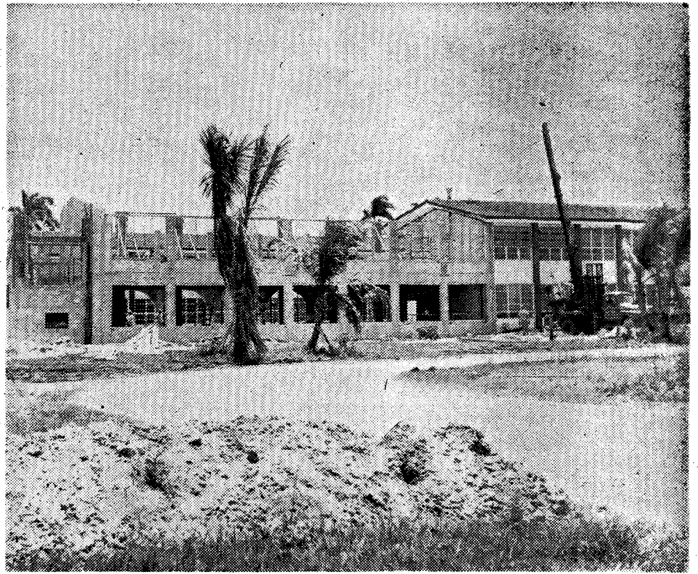
NEW ADDITION to St. John Vianney Minor Seminary is now under construction and is expected to be completed by September in order
