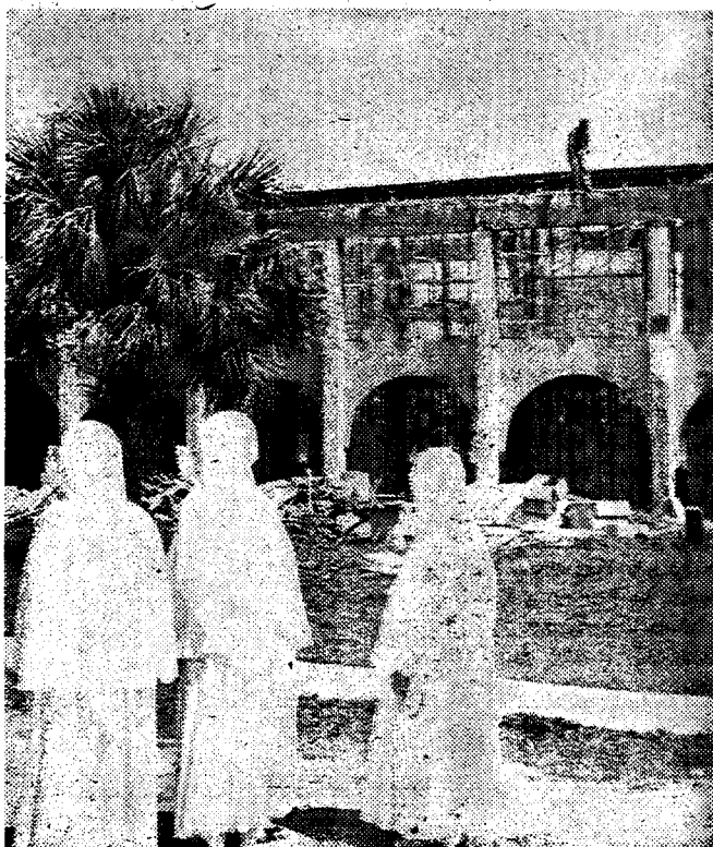
SECOND ADDITION to St. Brendan School provides four new classrooms for the elementary grades. Sisters of the Holy Family of Nazareth are shown viewing the new construction at the school which is located at Galloway Rd. and SW 30th St.
