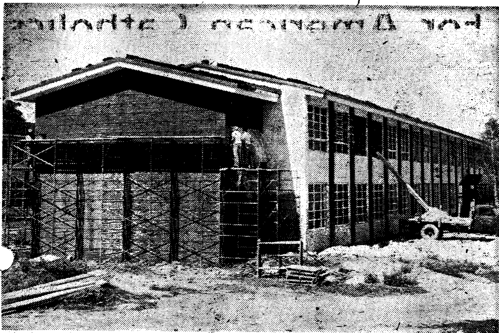
TWO-STORY addition to St. John Vianney Minor Seminary provides a large study hall, book room, perfect's office, large dormitory and
