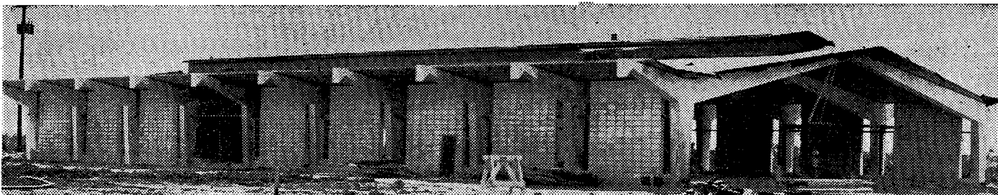
ST. GREGORY CHURCH in Plantation is now nearing completion. Constructed of reinforced concrete, the provisional church
