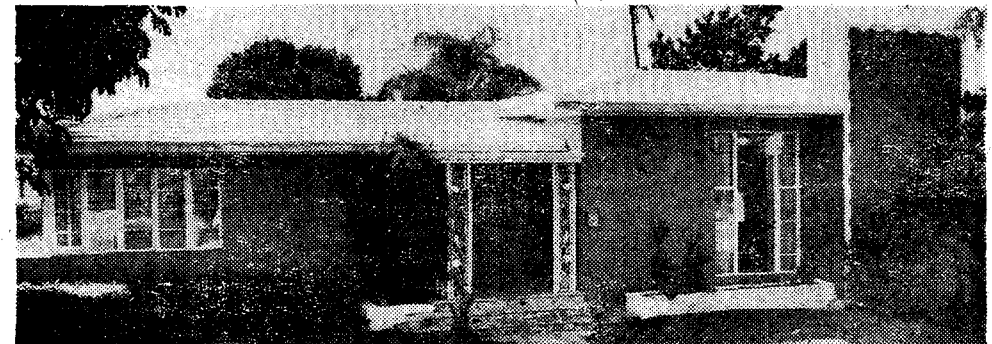
FLAT TILE ROOF on the home of Mrs. Gladys Hayden, 842 N.E. 96th St., recently was cleaned, sealed and coated
