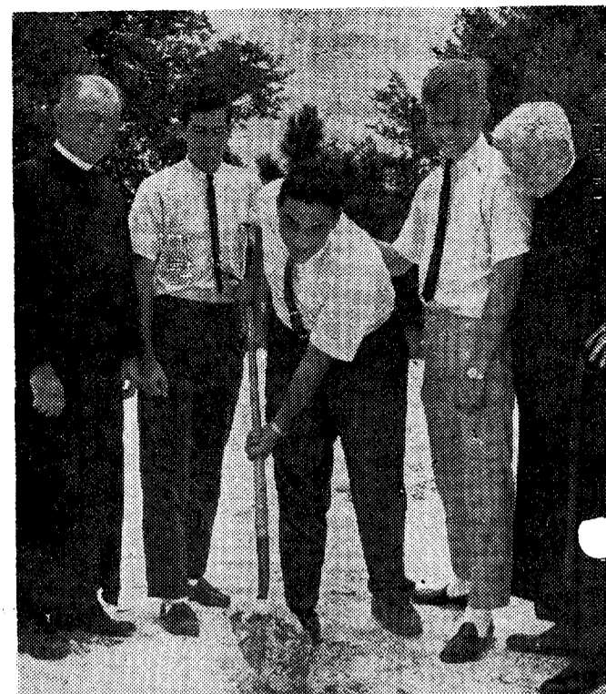
FIRST SHOVEL full of earth to break ground for a dormitory at Biscayne College was turned last week by Father Edward V. Stanton, O.S.A., former president of Villanova University, right, shown above with Father Edward McCarthy, O.S.A., college rector, and students Andrew Barrett, Louis Vitale, and Al Manning. The new building will cost about $450,000.
