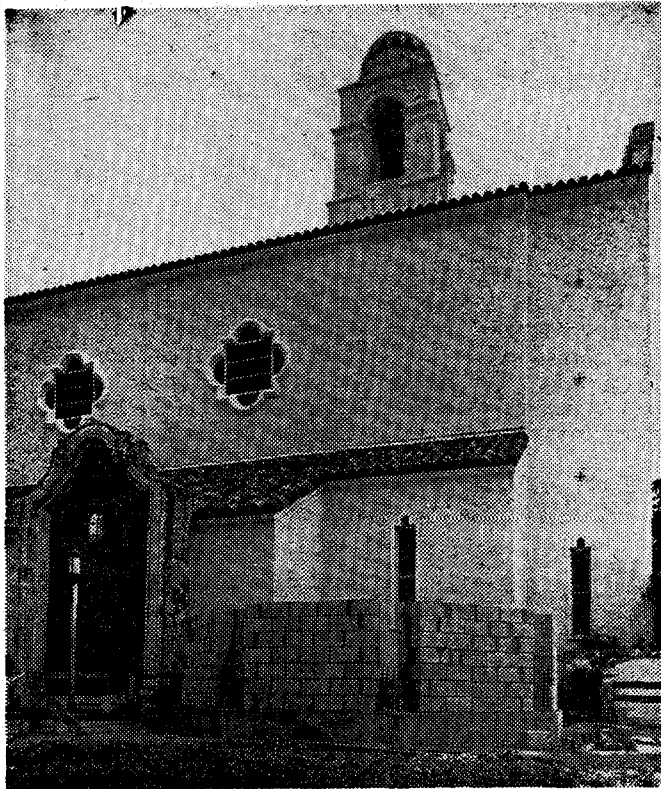
IF YOU'VE been wondering what is under construction near the front of St. Mary Cathedral, Miami, it's a new baptistry.
