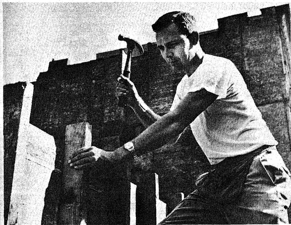
LEARNING the building trade from the ground floor up is Father Richard Becker, S.J., who is preparing for his assignment to a trade school in the Caroline Islands.
