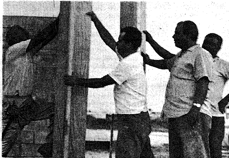
ON THE job training for seasonal workers learning carpentry is given by instructor George Sullivan, left, at a work site which, when completed, will be part of a training center for exceptional children.
