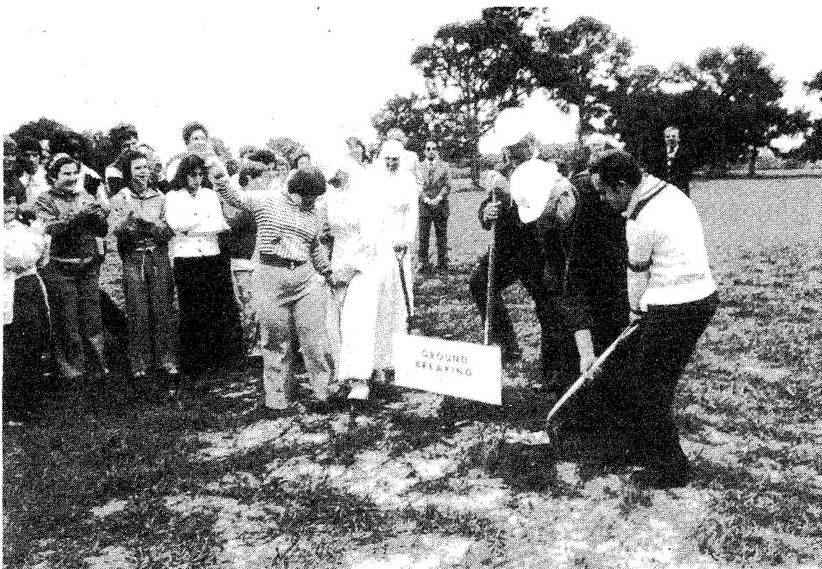
Encouraged by the applause of their school mates, Suellen Scott and Jeffrey Stephens, aided by Sister Lucia, director and Archbishop Edward McCarthy, speared the first shovelfuls of earth on the site of the new Industrial Arts building at the Marian Center school for retarded children. The new service will provide training skills for young adults preparing them for outside work. Susie and Jeff were honored at the groundbreaking ceremonies as the first students of the newly established school in 1964, for special education.
