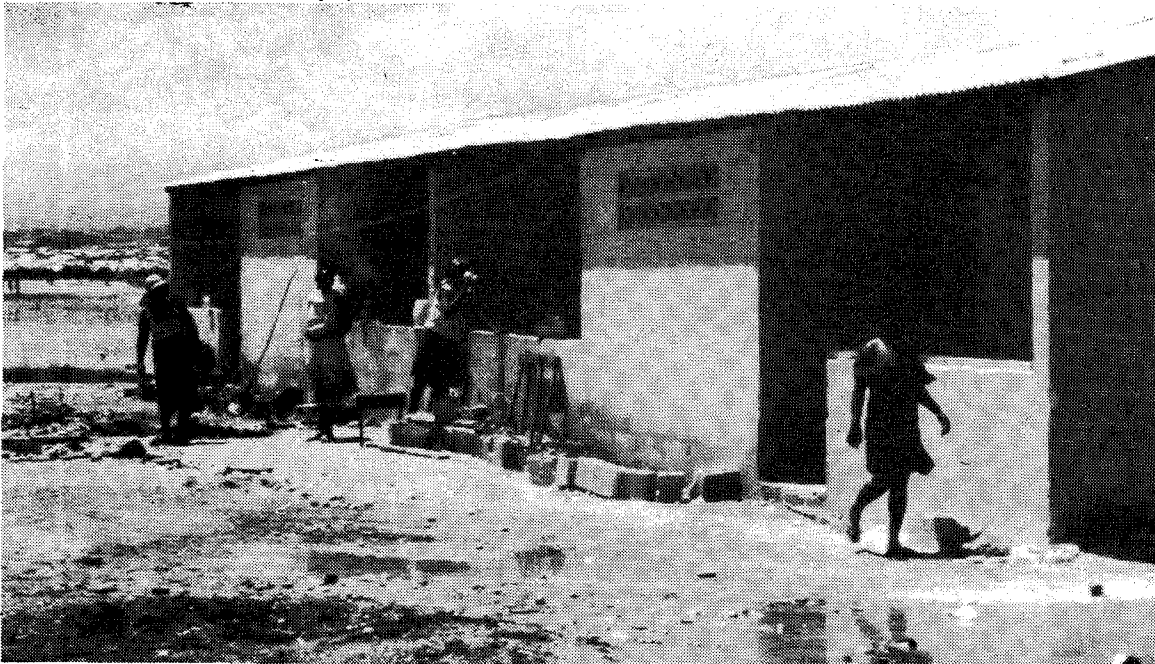
NEW HOMES FOR HAITI— This is one of 78 new housing units being constructed for the poor of Port-de-Paix, Haiti, by the Miami lay organization Amor en Accion (Love in Action). Since the families themselves provide the labor, cost of a unit runs between $250 and $300 for cinder block and other materials. A school and vocational center also are being built.
