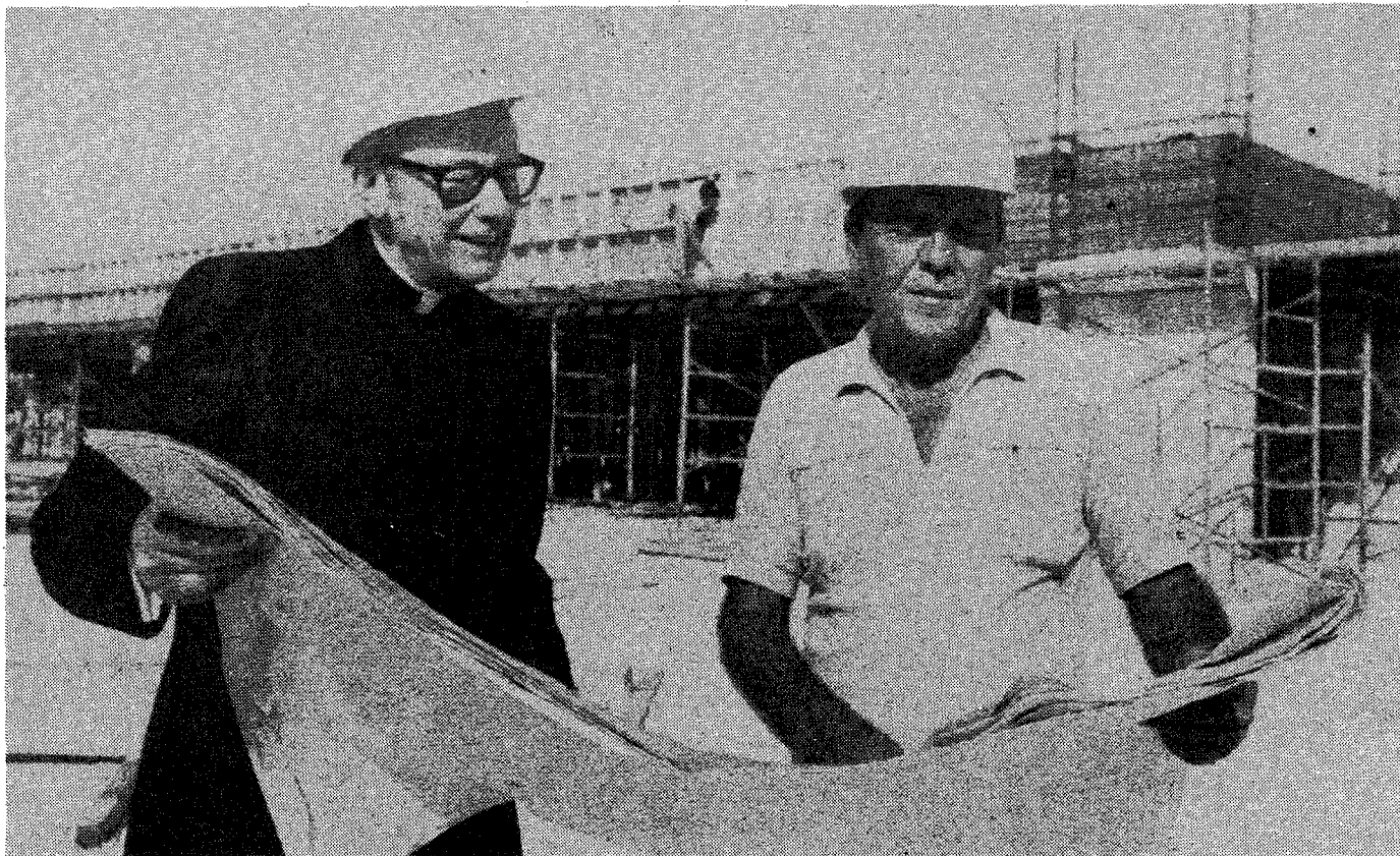
Archbishop McCarthy and Bill Hines, supervisor of the construction, talk over plans for the building, underway.
