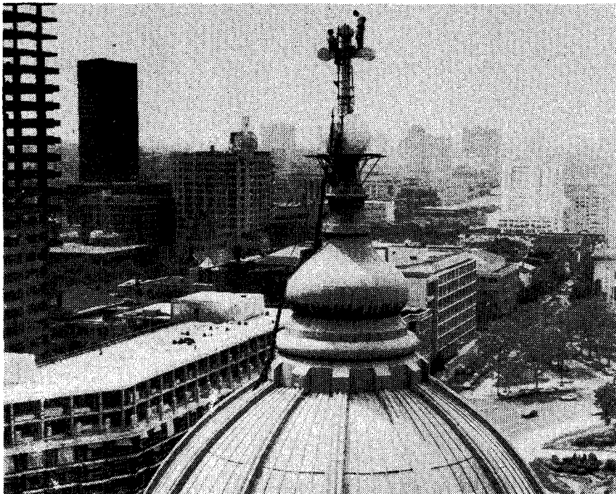
CROSS PURPOSE — Steeplejacks Frank Kenney and Joe Broderick put one of seven coats of paint on the cross atop the Cathedral Basilica of SS. Peter and Paul in Philadelphia. The men will top off the job with an application of gold leaf. The workers are employed by Jack Hassler Steeplejacks, the company that first worked on the dome in 1911.
