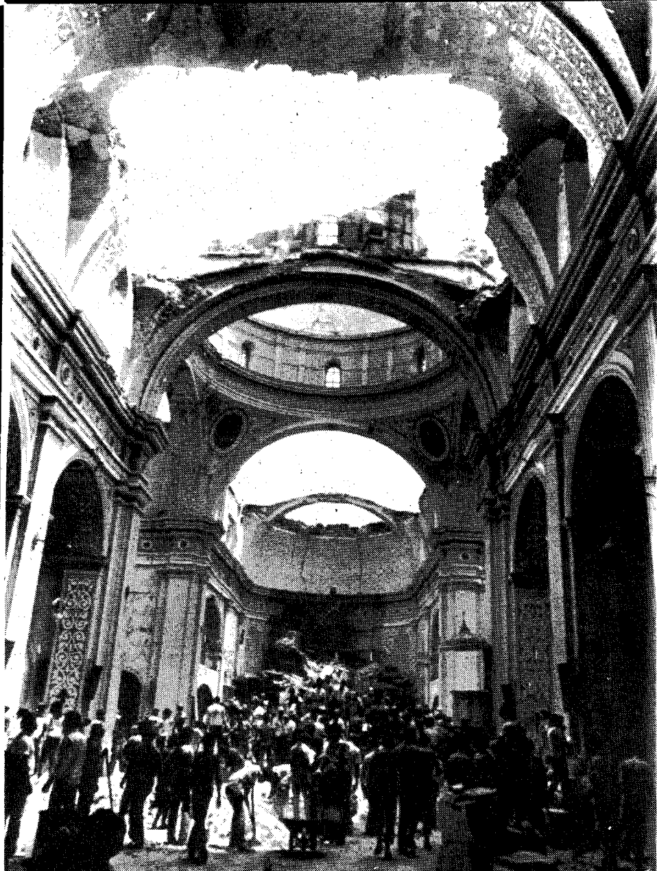
COLOMBIAN QUAKE - Workers attempt to clear the rubble left by an earthquake which wrecked the cathedral in Popayan, Colombia, on Holy Thursday, burying many worshippers. Pope John Paul II sent condolences to families of the victims. (NC photo)
