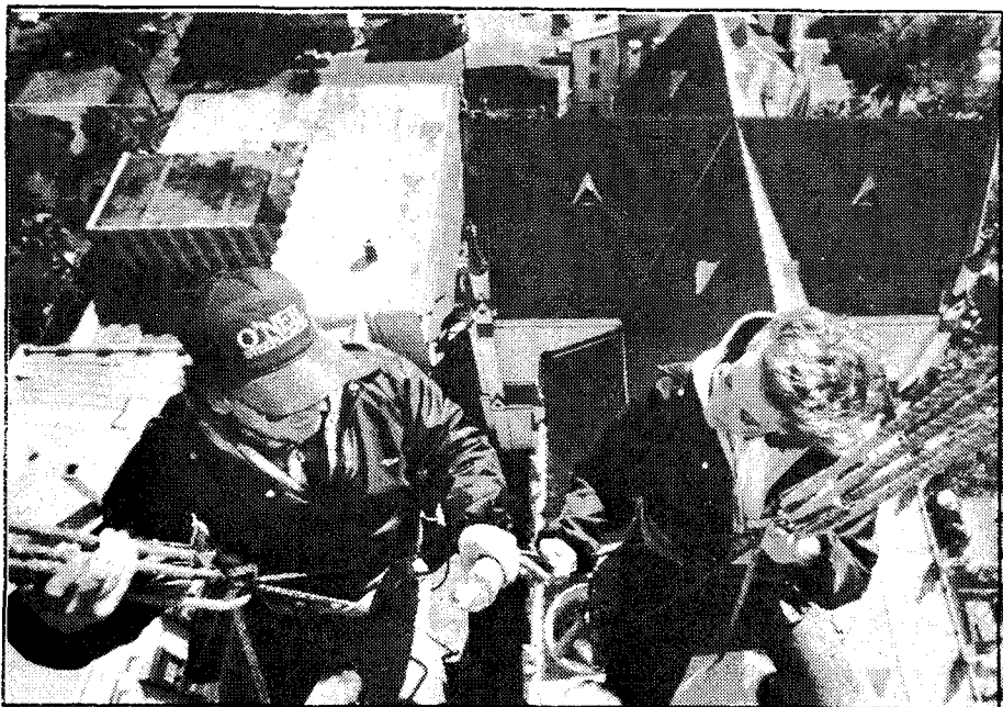
Steeplejacks Tim and Linda O'Neil repair the steeple of St. John the Baptist Cathedral in Savanna, Ga. The couple is part of a family that travels the country to repair the roofs of churches and other buildings. (NC photo by Darrell O'Neil).
