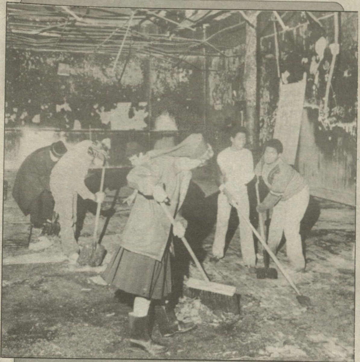
If we see only the evil in any situation (such as this building ravaged by fire), then there is much that has been missed, writes Blessed Sacrament Father Eugene LaVerdiere. One should look again. (CNS photo)
