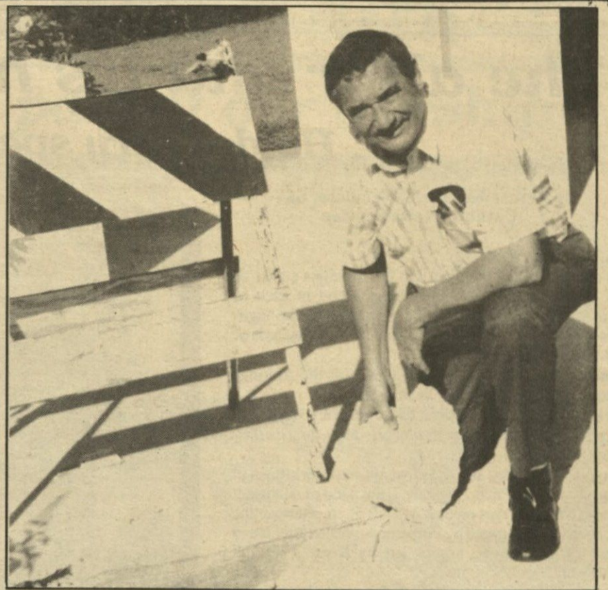
ACT OF GOD--David Pyle, Plant Manager of the Archdiocesan Pastoral Center, holds one of several chunks of concrete that were blown out of the foundation of the Papal Cross when the cross was struck by lightning recently. Observers were reminded of how lightning caused the Mass at Tamiami Park to be discontinued by the Pope when he was here in 1987. The 75-foot cross, transplanted from the park to the Pastoral Center three years ago, acted like a lightning rod and was unharmed.
